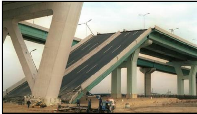
Figura 12. Colapso de una sección del puente Nishinomiya 1995 (Obtenida de: https://www.researchgate.net/figure/Collapse-of-a-section-of-the-Nishinomiya-in-1995-M-w-68-Hyogoken-Nanbu-earthquake_fig5_272971872 )
