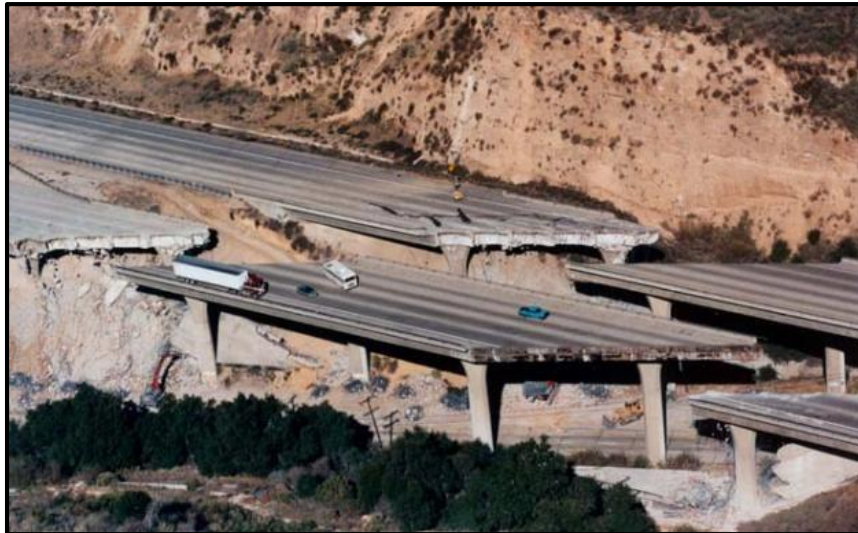
Figura 3. Colapso del paso a desnivel Gavin Canyon. (Obtenida de https://co.pinterest.com/pin/146718900334095793 )
