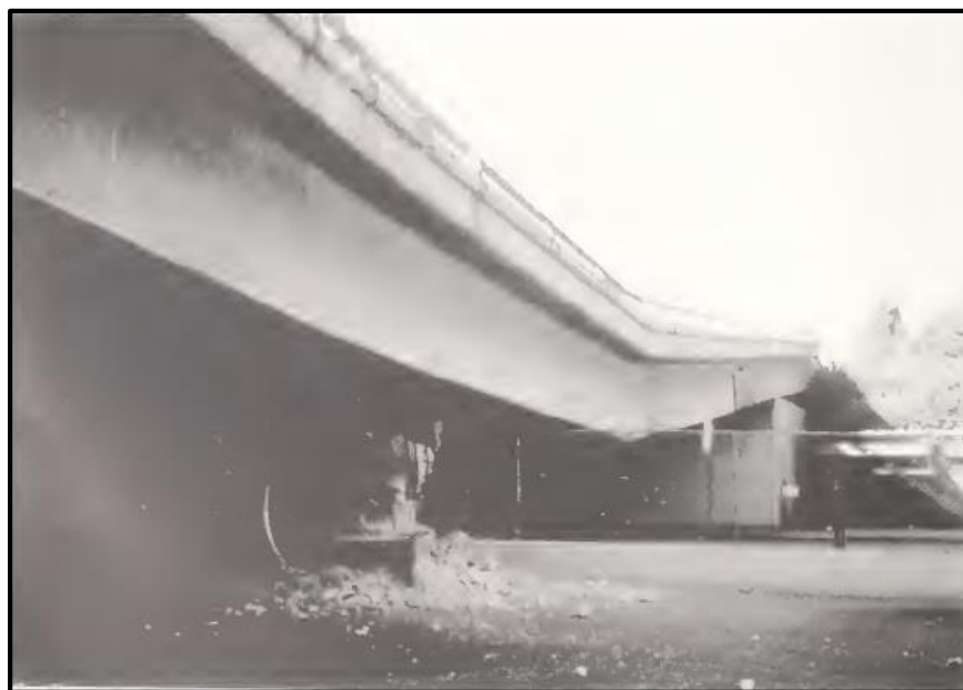
Figura 10. Colapso del Vano del puente sobre la Avenida Fairfax (National Institute of Standards and Technology, 1994)
