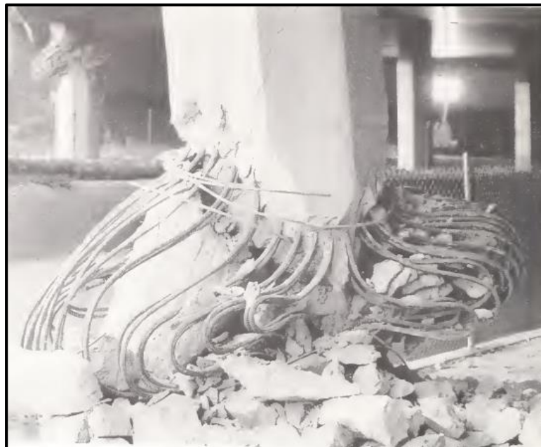
Figura 8. Daño al Pilar del puente "Bull Creek Canyon Channel" (National Institute of Standards and Technology, 1994)
