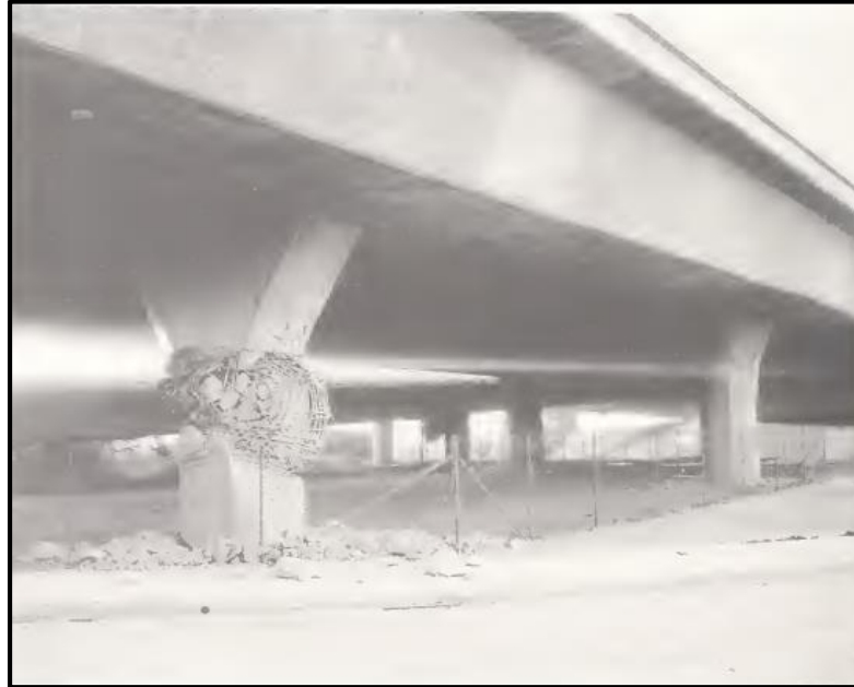
Figura 7. Daño a pilar en el cruce a desnivel Mission – Gothic (National Institute of Standards and Technology, 1994)
